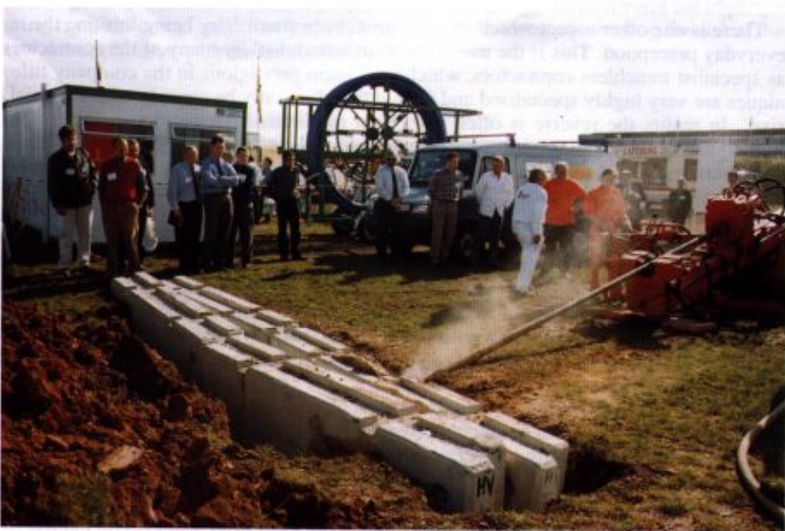
Powermole/SE's PM903 Dry-Rock Drilling Rig as demonstrated at the UK No-Dig Live 98, drilling through 2 x 450 mm steelmesh reinforced concrete motorway lane barriers.
