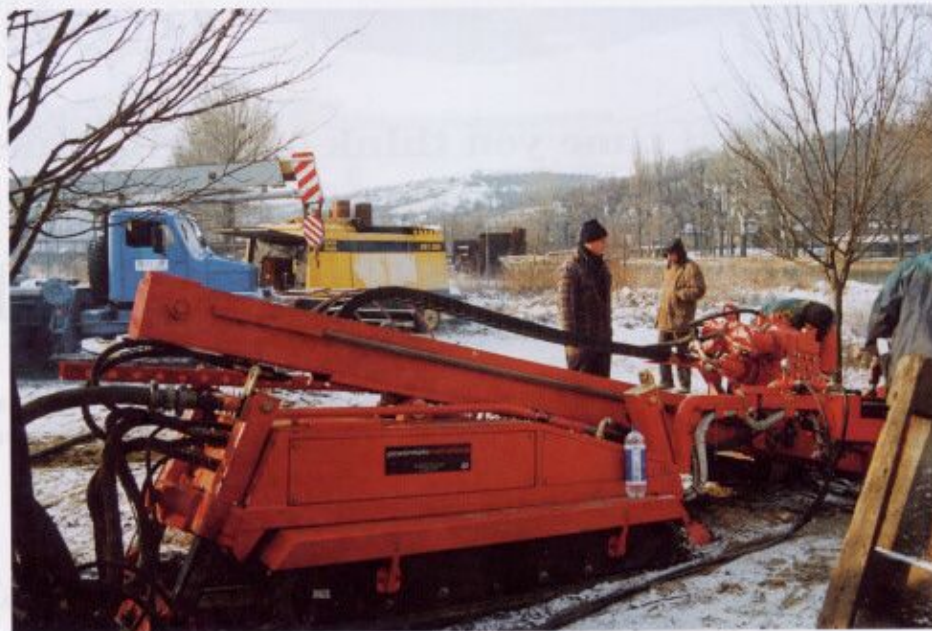
The PM903 rig drilling under the River Morana at Napajedla, Czech Republic.
